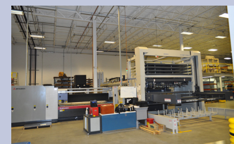
View of Laser and Material Tower
